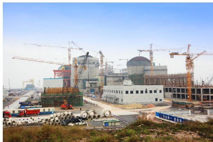
Figure 2.18 Hualong-1, HPR-1000, Fangchenggang 3 and 4
